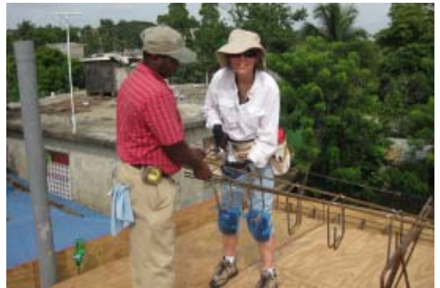
Elaine New uses a “twister” to attach wire around steel rebar as she helps to build a church and school in the Dominican Republic earlier this summer.
